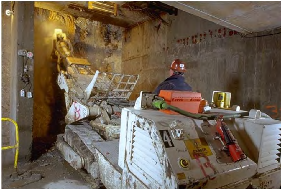
Figure 12-5 Excavation of the Frozen Ground at the Front of the Tunnel Shield by Roadheader
