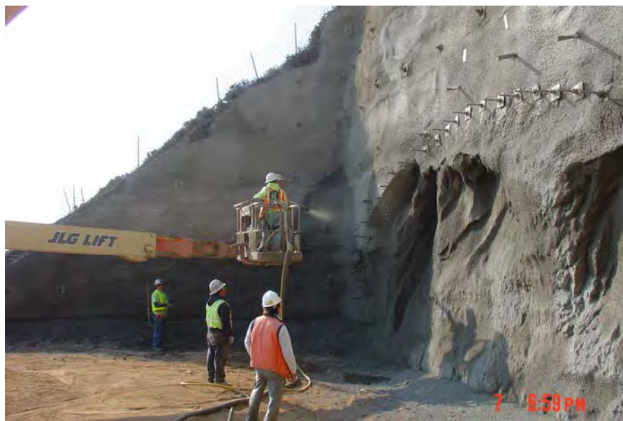
Figure 9-18 Pre-Support at Portal Wall and Application of Shotcrete for Portal Face Protection (Devil's Slide Tunnels, California)
