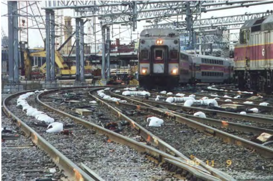
Figure 12-12 Ground Freezing System in Operation while Commuter Trains Run Through the Area
